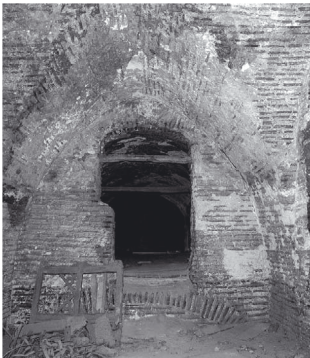
Fig. 5 Cross-vaulted room above the exonarthex of the church, opening into the long room above the atrium (seen from east)
