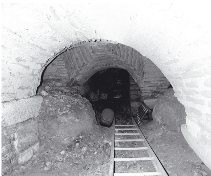
Fig. 4 Cross-vaulted substructure beneath the antechamber of the Large Hall, view from east. The two re-used piers supporting the vaulting can be seen on the right. On the left, the sixth-century substructure wall of the demolished triple arcade between the antechamber and the Hall (up to the level of the large stone blocks)
